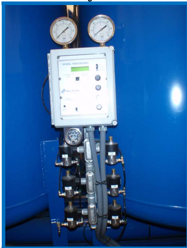
Controller and solenoid valves
