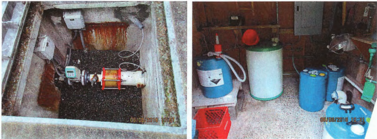
Figure 4. (Left) Vault with the raw water flow meter, sample tap, and chlorine injection line. This meter controls the chlorine injection. (Right) Hypochlorite disinfection treatment plant with NSF certified hypochlorite, hose for make-up water, 3 parts water and 1 part 12.5% sodium hypochlorite, flow paced peristaltic feed pump.
