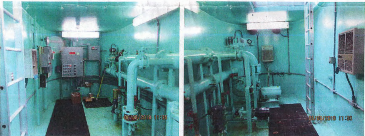
Figure 12. 520 BPS. Below grade vault. No backup power generator. Constant run pump station. (Left) Booster pump controls, cla-valve, flow meter, two 3/4hp pumps. (Right) 5hp pump, 50hp pump.
