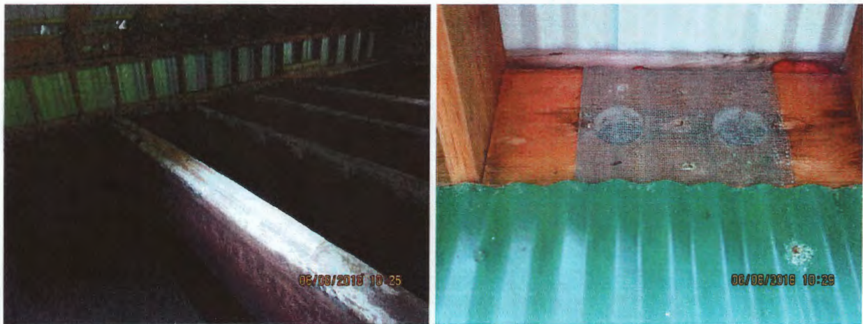
Figure 5. Baffled chlorine contact tank. (Left) View from the vertical access hatch. Purple manganese staining. (Right) Overall good screens and seals. Please double check the seal between the walls and the roof.
