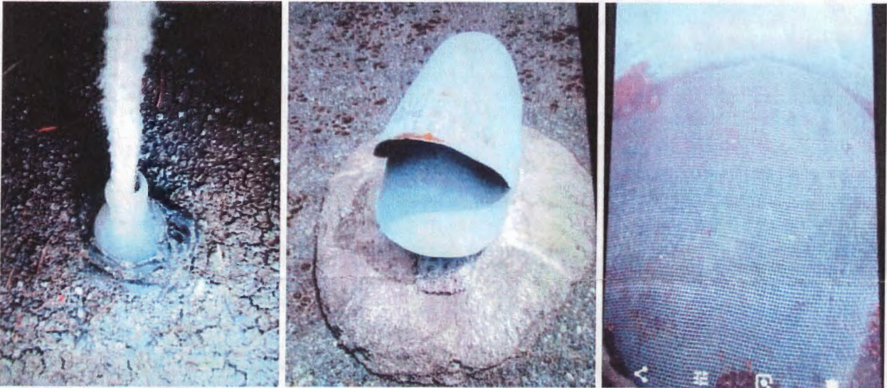
Figure 11. (Left) Level indicator cable is covered with the metal tent. The cable enters the roof through the rubber fitting. (Center) Air vent design allows debris to collect on the horizontal screen underneath. (Right) Air vent screen. (Photos provided by the Association during the survey).
