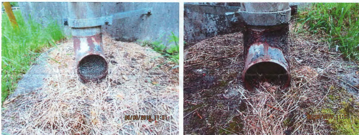
Figure 10. Storage tank overflows with screen (maybe 4-mesh). Overflows need 24-mesh screen to prevent insects from entering the tank. Ideally, there is an airgap.
