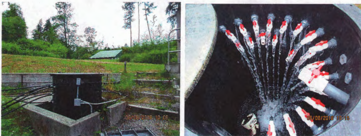
Figure 3. Collection chamber. (Left) Overview showing the black pipes from the wellpoints entering the collection chamber. The retired upper reservoir is in the background. (Right) Inside the collection chamber. The screened overflow (not 24-mesh) goes to a dedicated vault that overflows to the hillside (not shown here).
