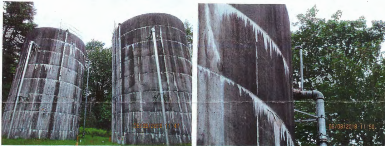
Figure 9. North and South storage tanks. Float control tank level controls Dockton Springs by radio transmittance. No pressure transducer. (Left) Overview. (Right) Vent on the overflow pipe.
