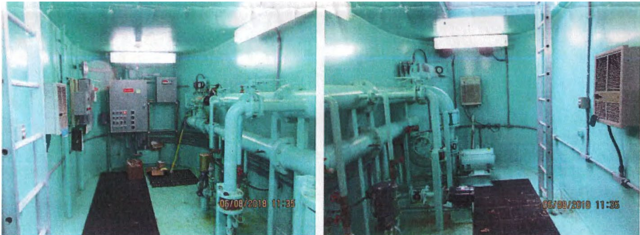
Figure 2.10 520 Zone Booster Pump Station
