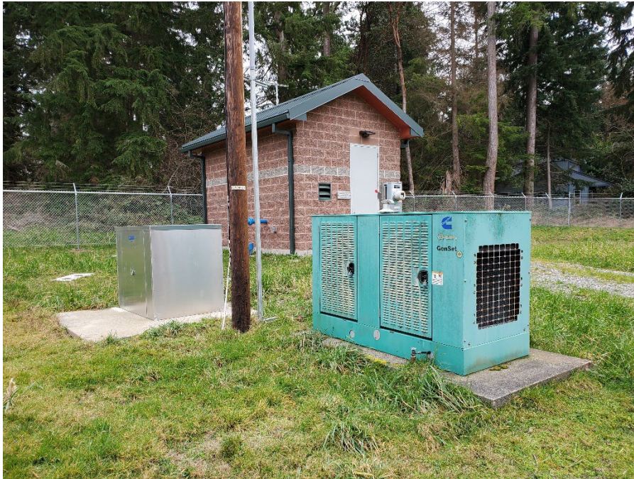
Figure 2.6 Sandy Shores Well Enclosure, Generator, and Treatment Building
