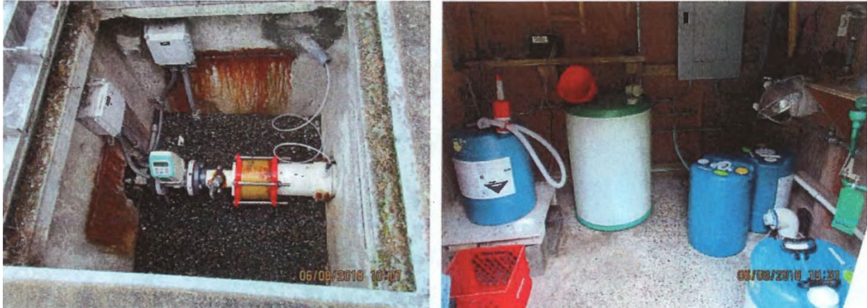
Figure 2.4 Raw Water Flow Meter and Chlorine Treatment Room
