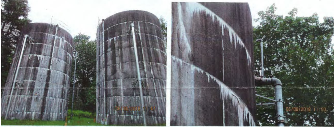
Figure 2.8 North and South Storage Tanks
