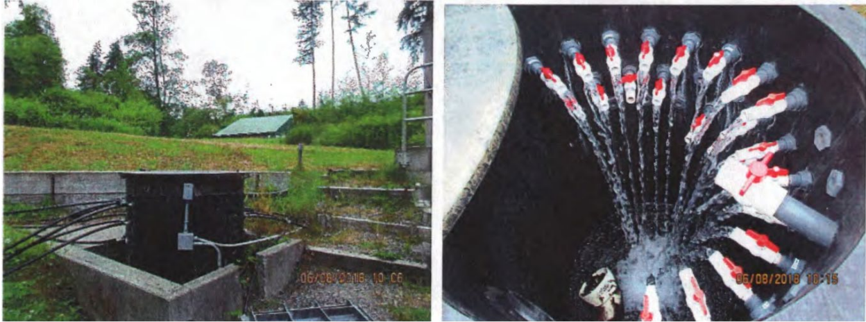
Figure 2.3 Dockton Springs Collection Chamber
